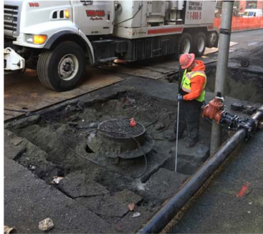
Excavating, using a vacuum truck, to expose and verify water services on 1st Ave S
