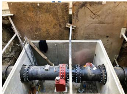
Vault installed on 1st Ave S just south of S Main St. This vault will house a valve for the new water main.
