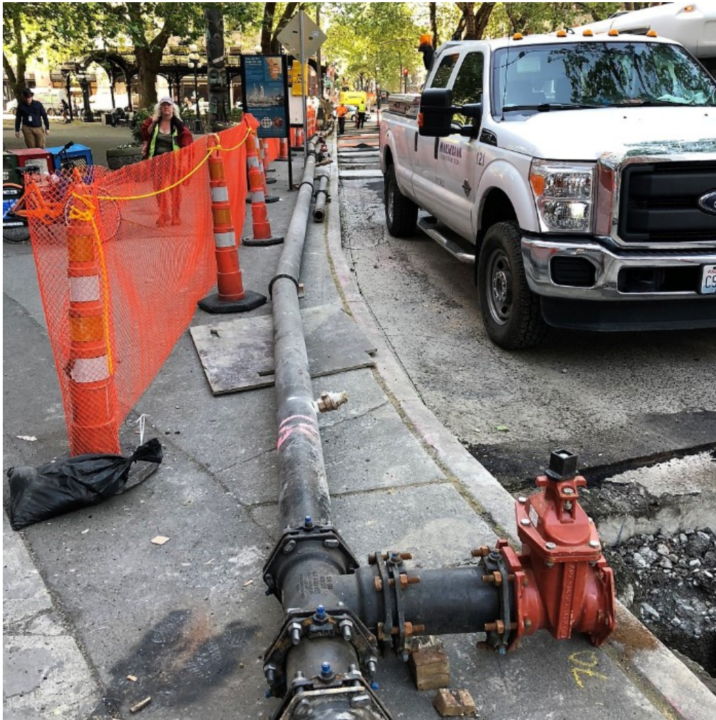
Installing the temporary water main on 1st Ave between Yesler Way and Cherry St.
