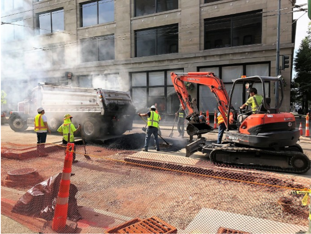
Installing asphalt paving on S Jackson St just east of 1st Ave S.
